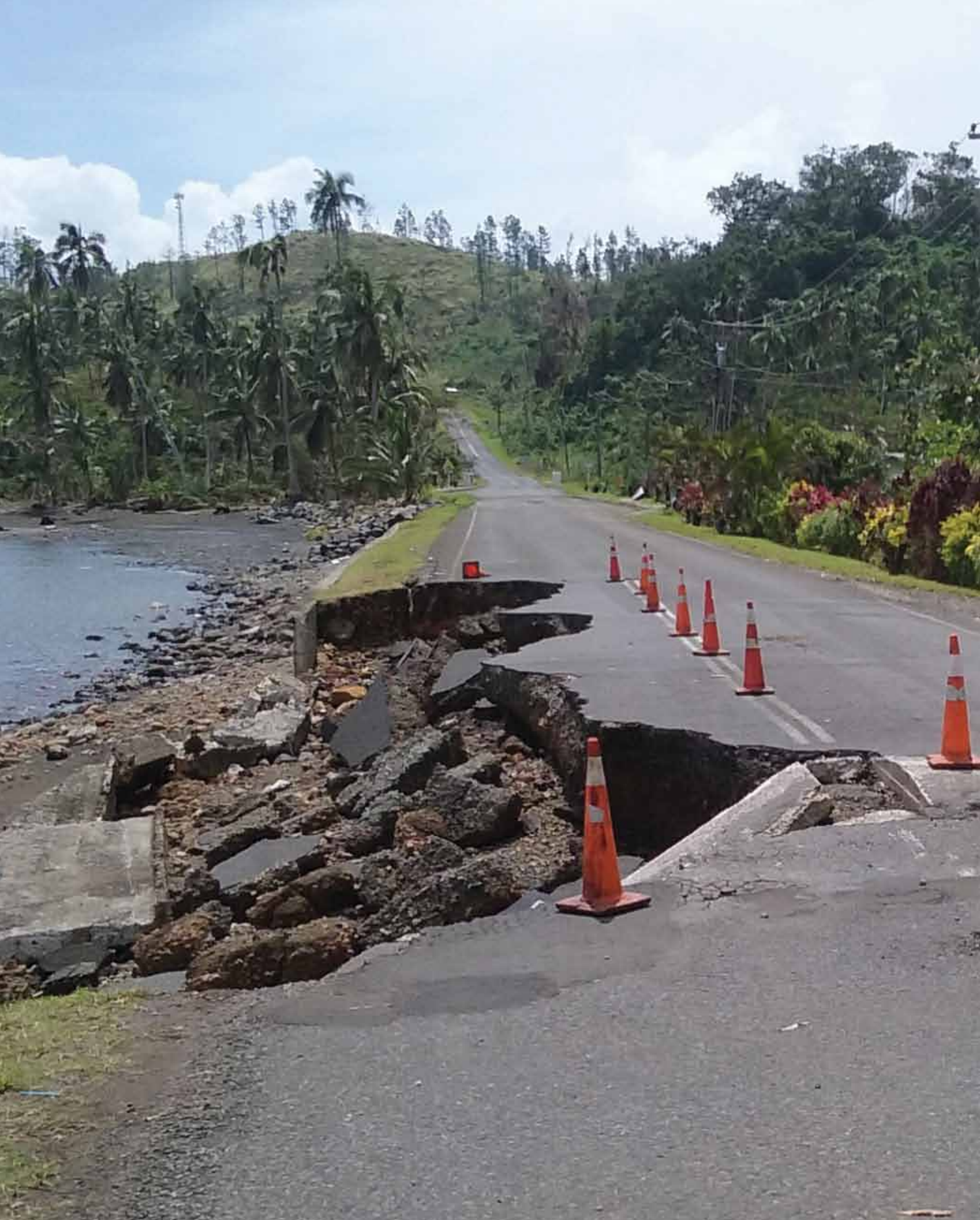
Damage to roadway in Cakaudrove Province on Vanua Levu Source: Ministry of Infrastructure
